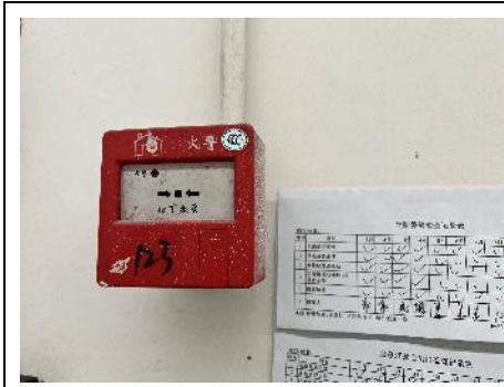
Fire alarm button
